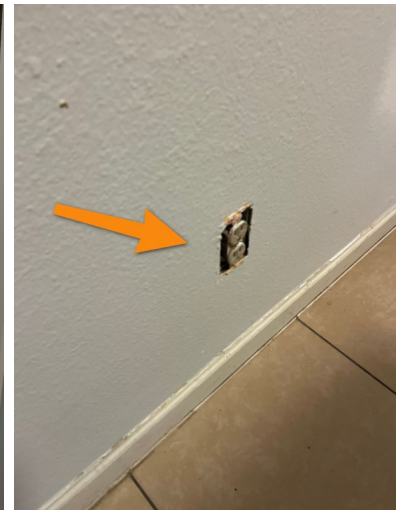
Unit A Kitchen
