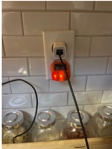
Unit A Kitchen
