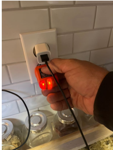
Unit A Kitchen
