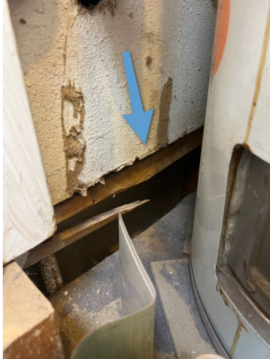
Water Heater Closet B
