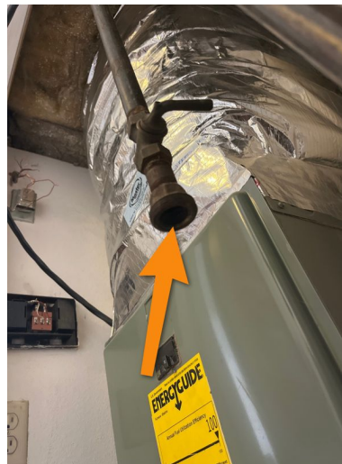
Unit A HVAC Closet,
