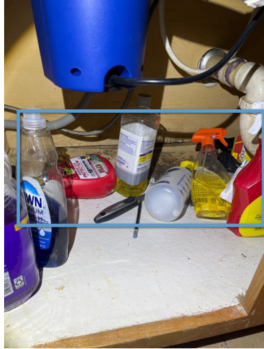
Unit A Kitchen
