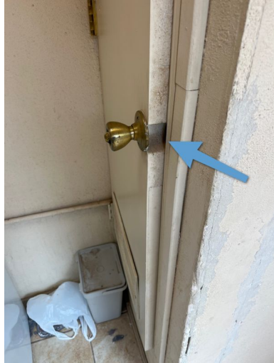
Water Heater Closet B
