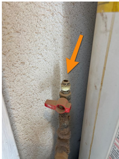
Water Heater Closet B
